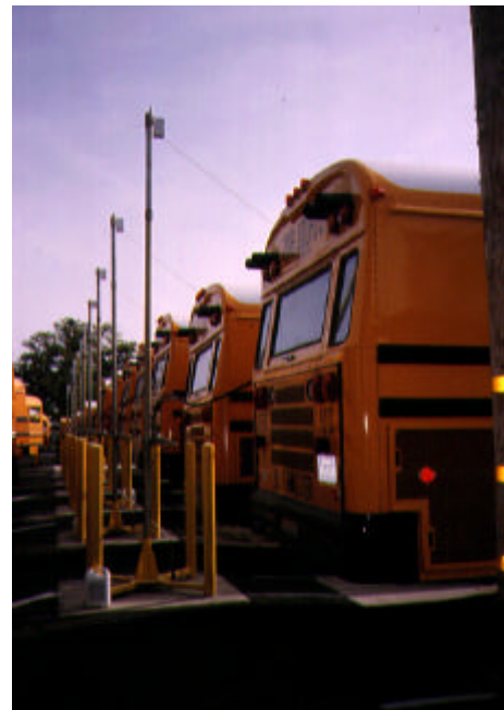
Natural gas-powered buses fueling at slow-fill CNG fueling facility. Courtesy of California Energy Commission. 1999.
